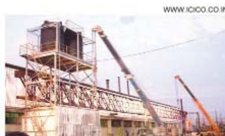
A 60-metre span lattice girder being erected for Automotive Axles Ltd in Mysore.
